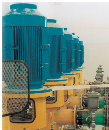
Mafraq Treatment Plant, Abu Dhabi
