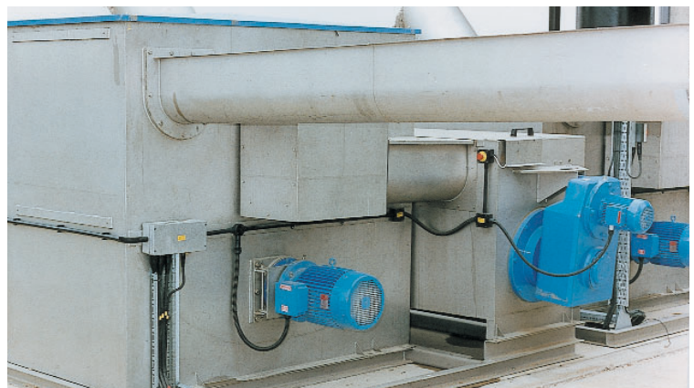
Bedford Sewage Works, Anglian Water Photograph courtesy of Jones and Attwood Limited
