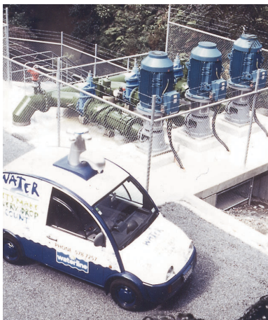
New Joyce Road Water Processing Plant, New Zealand
